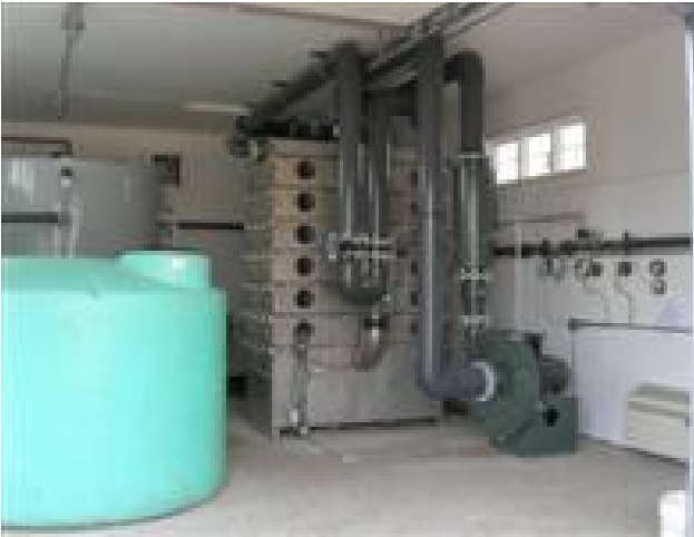
Air Stripping Tower & Blower Approx 8' Tall x 5.5' Square
